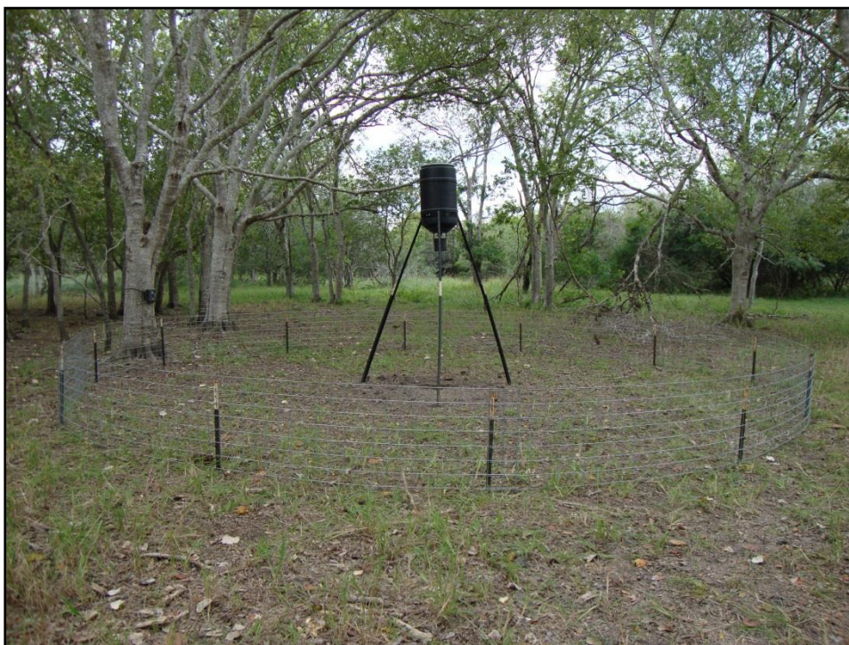
Figure 1. Exclusion fencing using 6 1.9-m livestock panels constructed into 9.4 m diameter perimeter circle around deer feeders with the aid of 12 t-posts in San Patricio County, Texas during the summer (29 June–28 July) and winter (5 November–3 December) of 2009.
